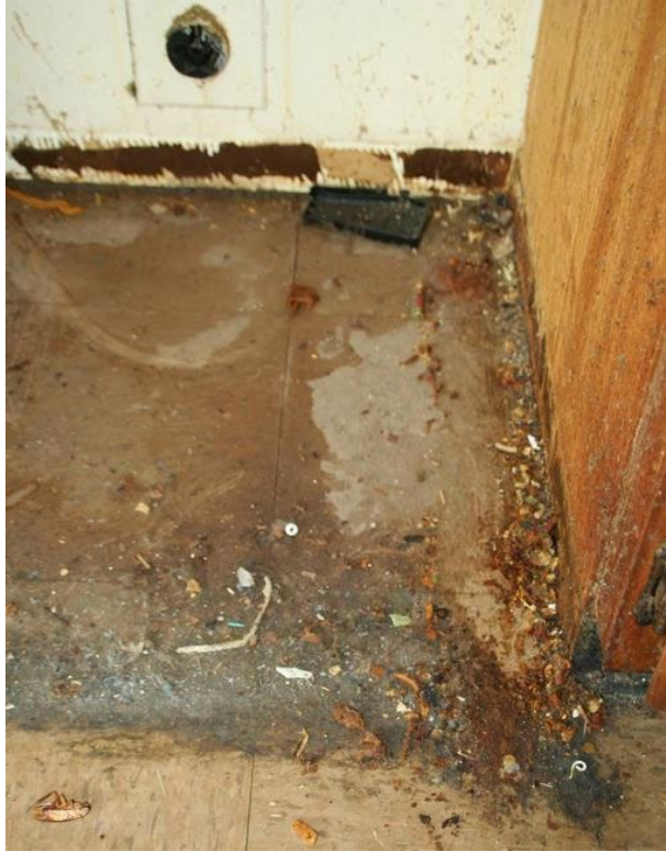
Figure 8. Evidence of American cockroach activity under a stove. (Photo: Liz Kasameyer).
