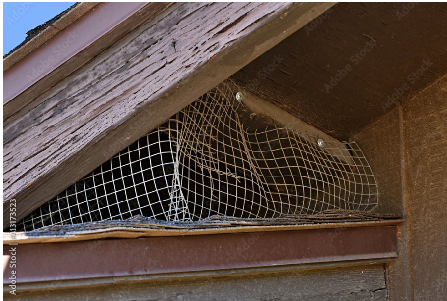
Figure 9. Pest-proofing is the best way to keep rodents out. Photo: Adobe Stock Images.
